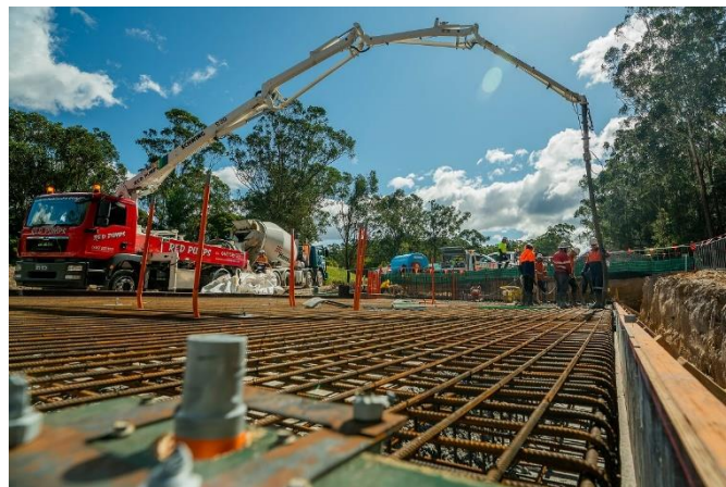
Image: Construction of the Valve Station Mardi Water Treatment Plant Valve Station
